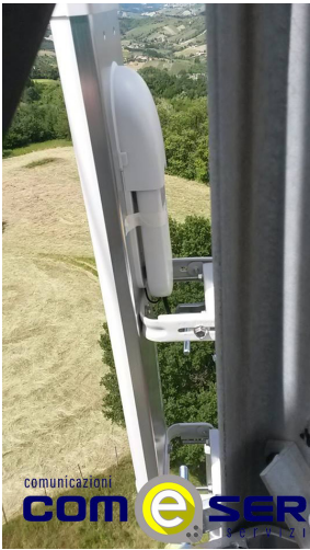
ePMP Access Point connects a community
