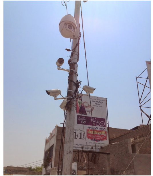
Cameras at intersection location
