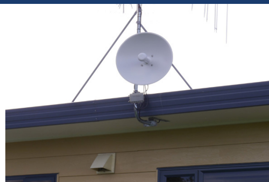
ePMP Force 200 connecting a residence
