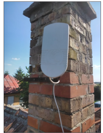
Station Module Provides Residential Connectivity
