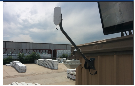
ePMP module and WLAN Access Point
