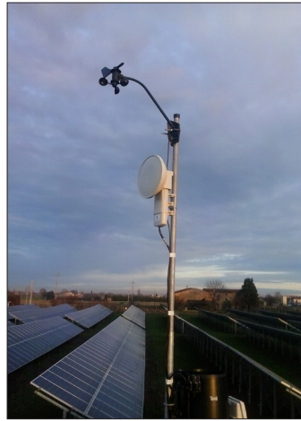
Collecting measurements and monitoring at a solar farm
