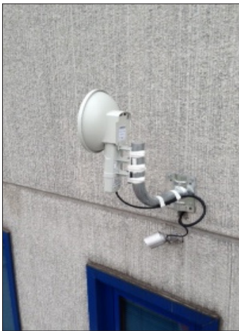
SM providing video surveillance at a business location
