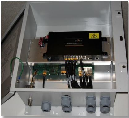
Figure 8 Cabinet (with switch)
