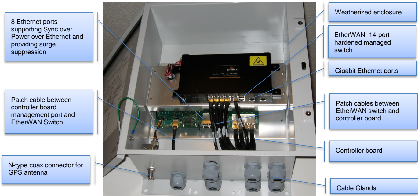
Figure 29 CMM4 internal view, including cable glands
