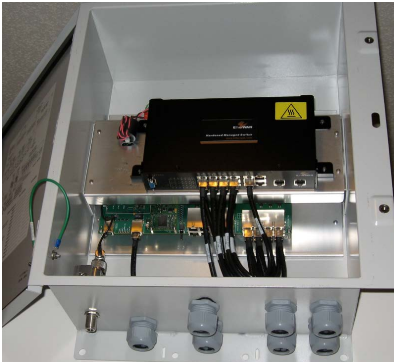
Figure 42 CMM4 (Cabinet with switch)
