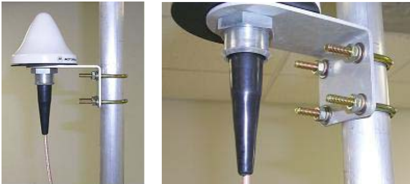
Figure 45 GPS antenna mounting
