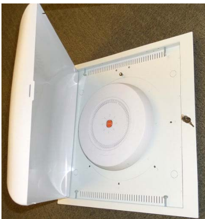
Indoor Enclosure, showing AP installed
