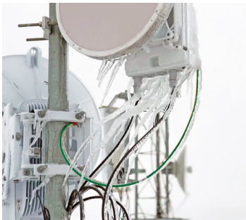
Cambium Networks' equipment is designed to withstand demanding outdoor environments.
